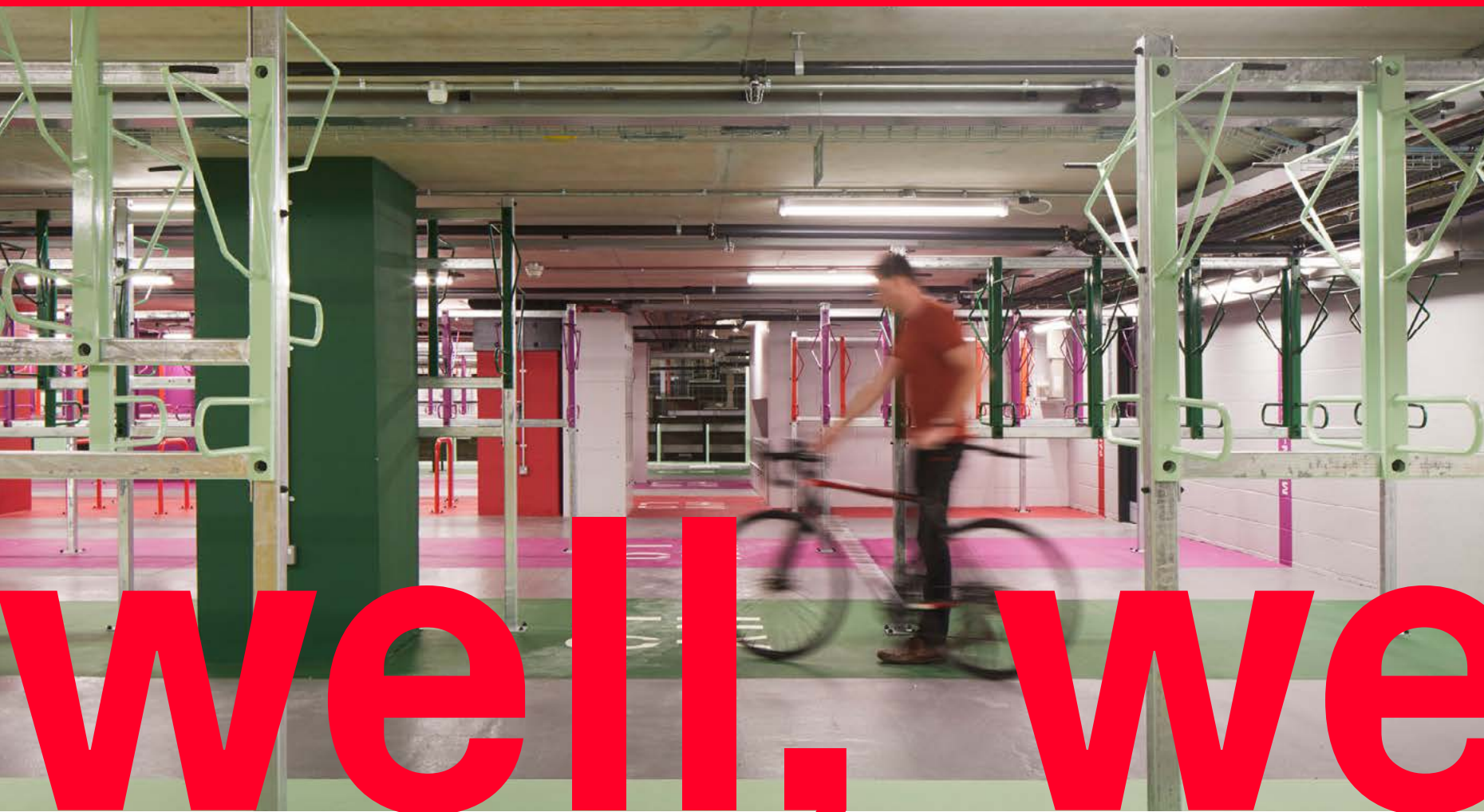
◀ Storage for 379 bikes including 76 Brompton Lockers in the basement
